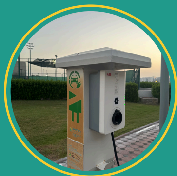
EV Charging Station
